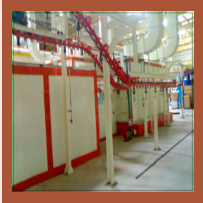
Conveyorised Paint Booths
