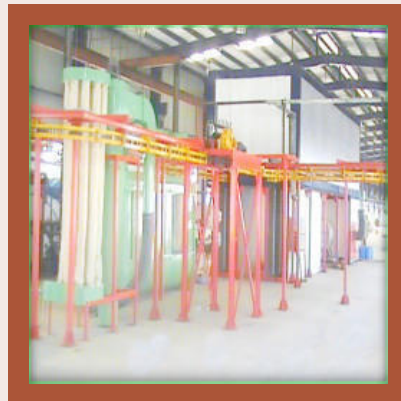
Conveyorised Powder Coating Plant
