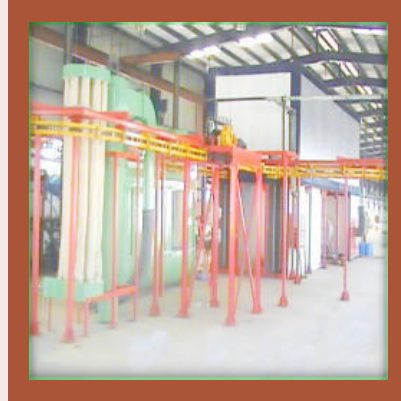
Conveyorised Powder Coating Plant
