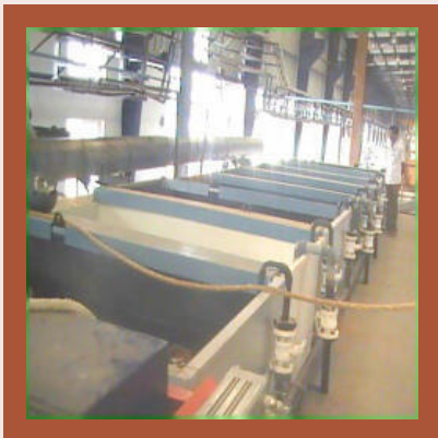
Batch Type Phosphating Plant
