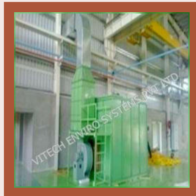
Activated Carbon Scrubber with Dry Type Paint Booth
