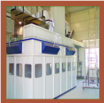
Clean Room for Paintshop
