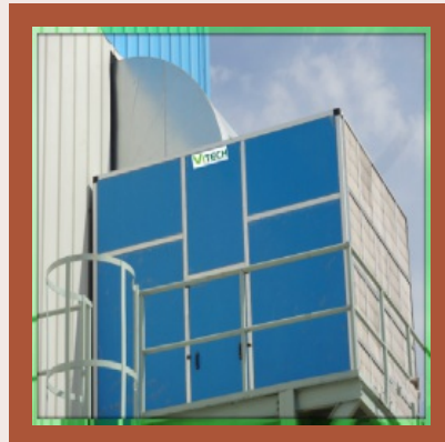
Air Handling Unit
