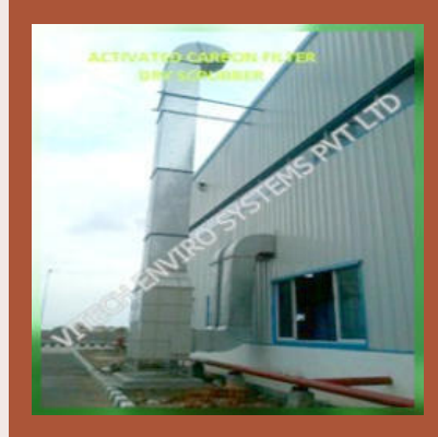
Activated Carbon Filter Dry Scrubber
